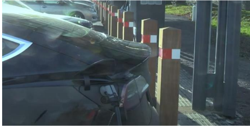
Bollards to protect EV chargers in South Gloucestershire's electric vehicle charging hub (source: https://www.youtube.com/watch?v=ODsnM9RY7_8 )
