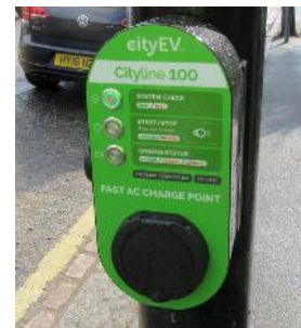
A City EV charging unit (source: www.autocar.co.uk )
