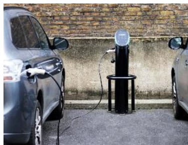
A Pod Point charger (source: www.current-news.co.uk )
