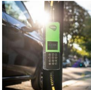
Closeup of an Ubitricity smart charging (source: www.electrive.com )
